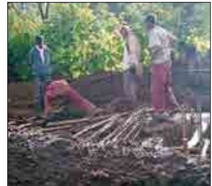
Construction started in earnest after the rainy season ended. Workers began laying out logs to cross muddy trenches.
